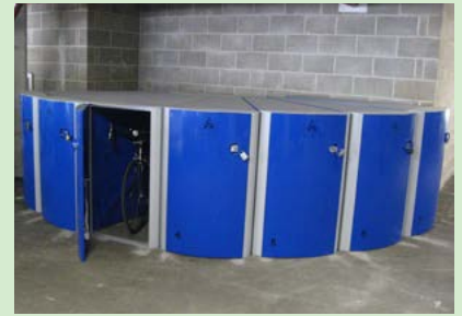
Seven Velo-Safe lockers were initially installed into the car park.
